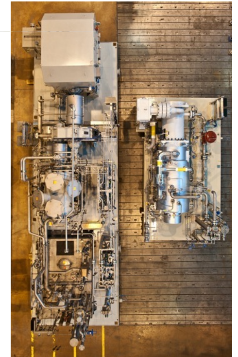
Conventional compressor train
