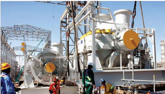
Compressor installation in 2006
