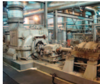
Process air compressor, compressor train.
