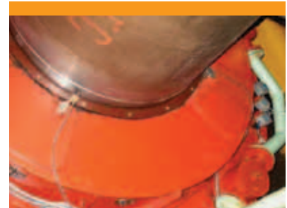
Figure 2: An example of XY transducer configuration where probes are connected to guide bearing cover.
