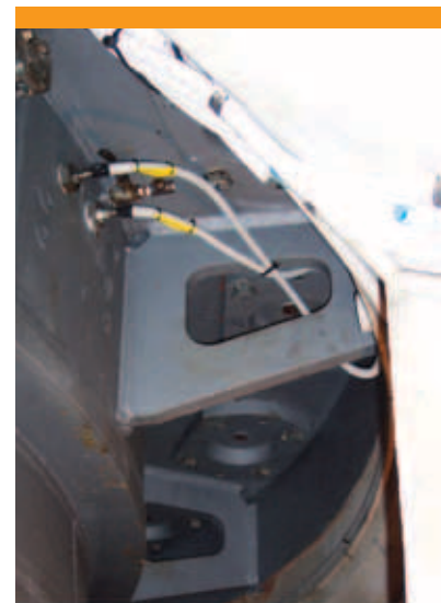
Figure 5: An example of redundant XY transducer observing shaft in the closed space (only one of XY transducer and its redundancy is visible at the photo)
